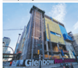
Glenbow Museum, circa 1976, undergoing extensive renovations, November 2023. Photo courtesy of Anthony Imbrogno.
