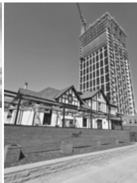
Future home of Elephant & Castle pub, formerly Davidson House (with 4th Street Lofts Tower in the background), August 2024. Photo courtesy of Anthony Imbrogno.
